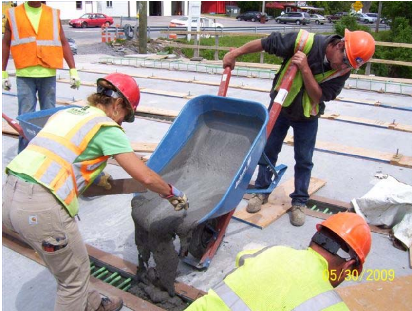
Figure 5. Field-casting UHPC on the State Route 31 Bridge over the Canandiagua Outlet in Lyons, New York. Photo courtesy of New York State DOT.
