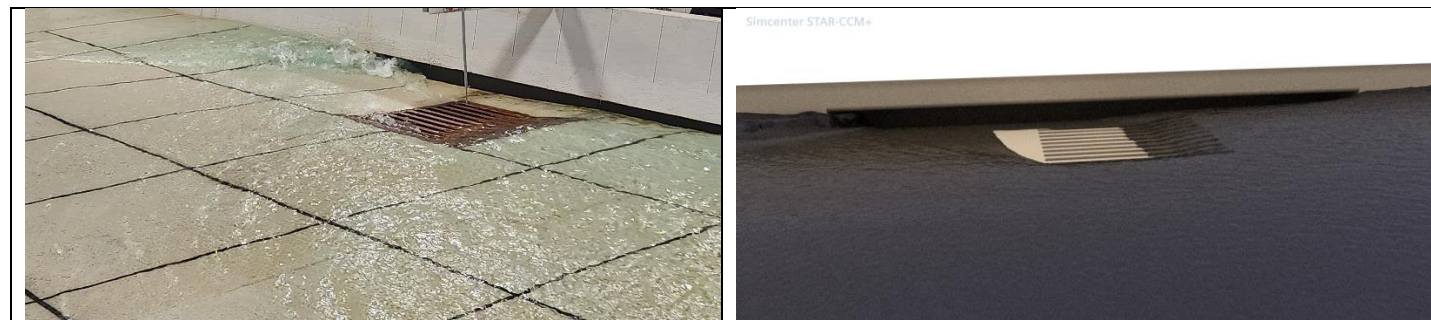
Figure 3. A similar portion of the grate is overtopped.
