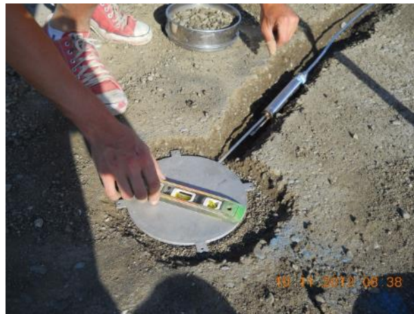
Figure 324. Photo. Installation of earth pressure cells for the two test sections - pressure cell on 670HC.
