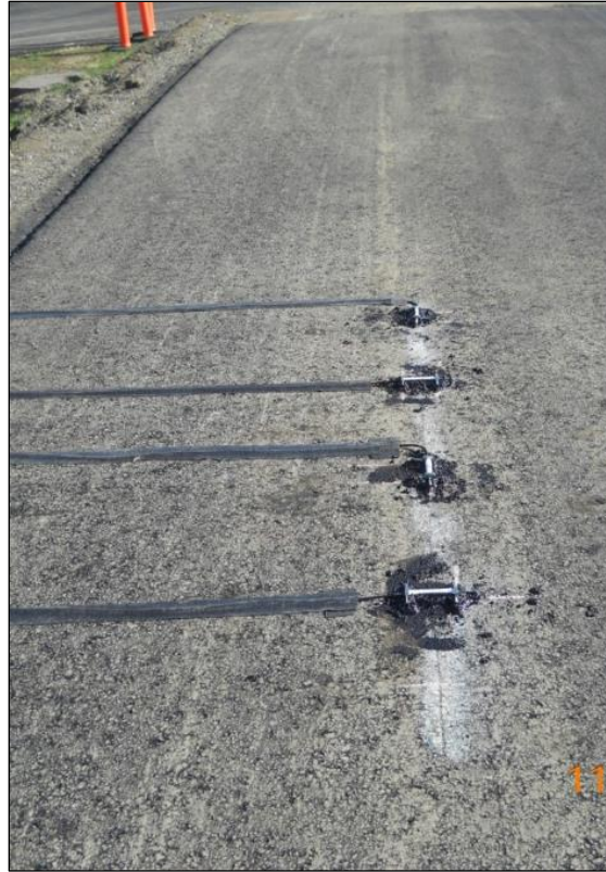
Figure 318. Photo. View of strain gauges and pressure cells installed on Section 671HC during construction - strain gauges on top of the bottom lift of AC.
