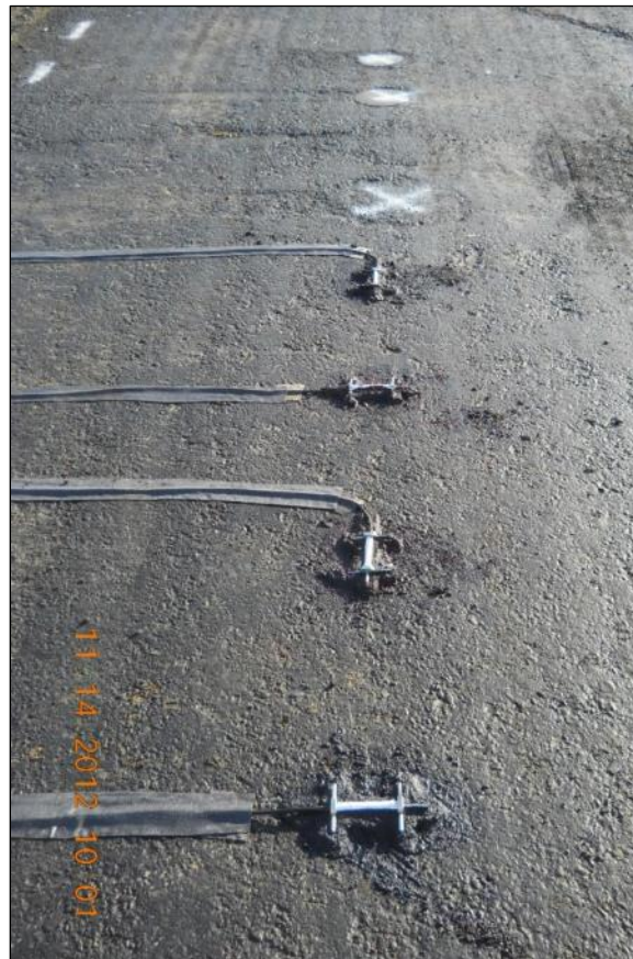
Figure 317. Photo. View of strain gauges and pressure cells installed on Section 671HC during construction - instruments on top of the recycled base.
