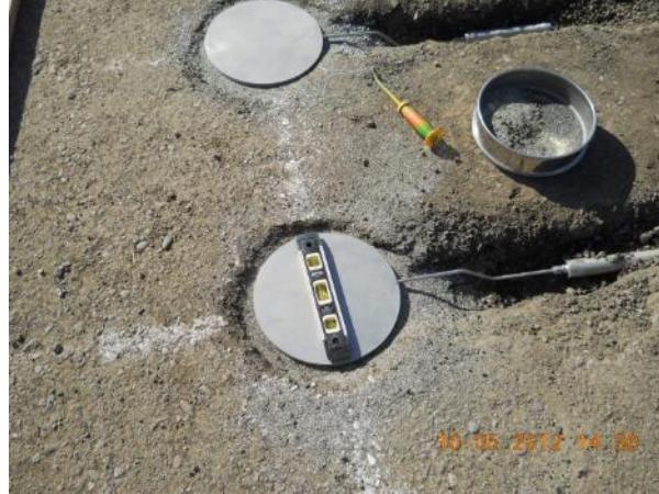
Figure 325. Photo. Installation of earth pressure cells for the two test sections - pressure cells on 671HC.
