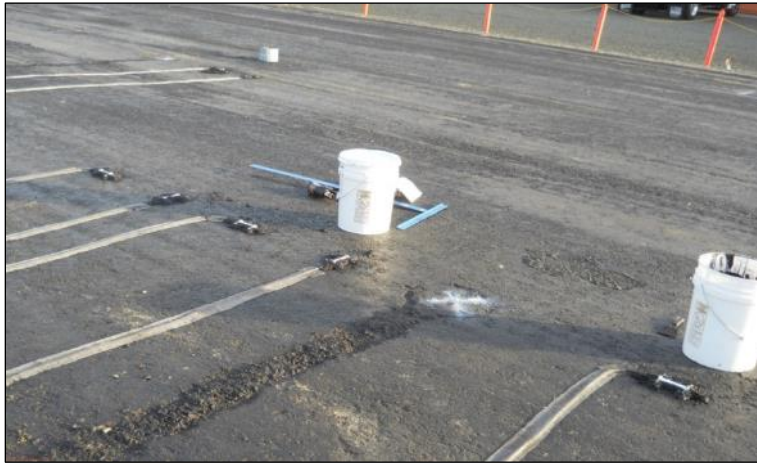
Figure 316. Photo. View of strain gauges and pressure cells installed on Section 670HC during construction.
