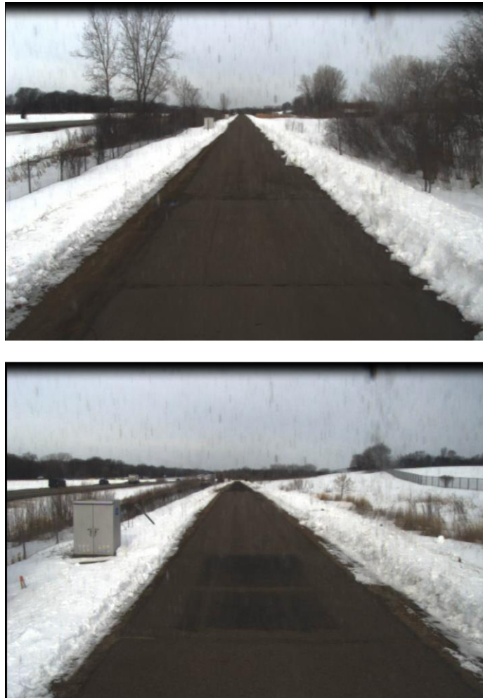
Figure 2. Picture of the road segment's road surface conditions
