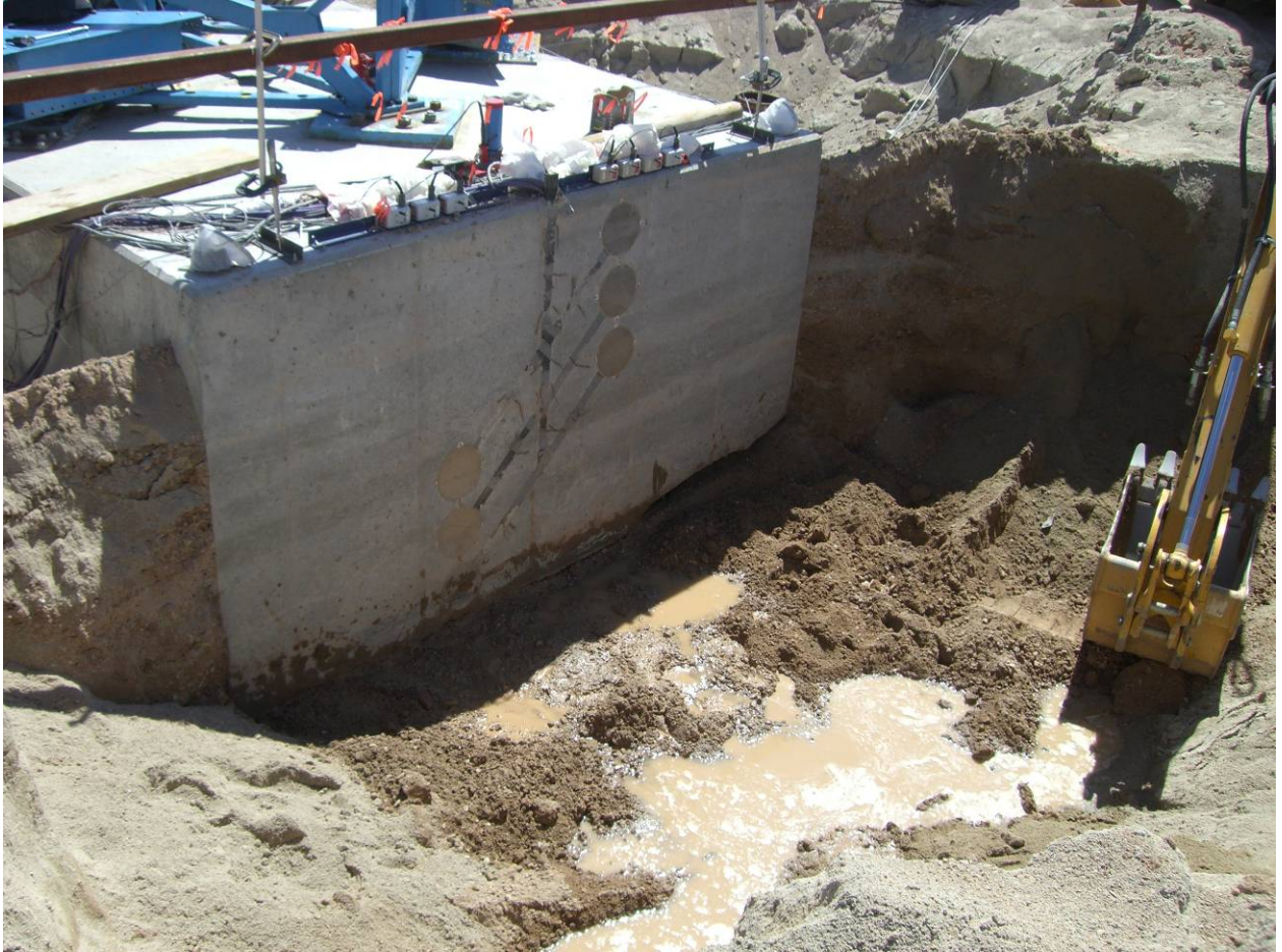
Figure 1. Photograph of front face of pile cap before backfill placement showing layout of six pressure plates.
