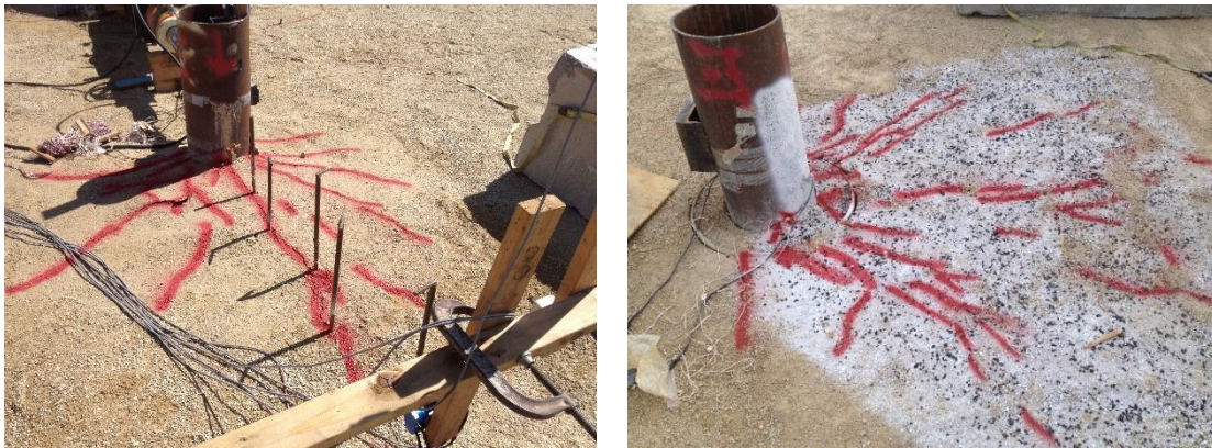
Figure 2. Surface shear cracks around a laterally loaded pipe pile (left) and CMS composite pile (right).
