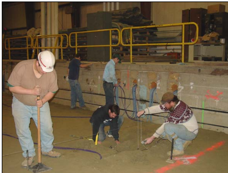
Figure 19. Instrumentation installation, showing a wire extended across the test basin for precisely locating sensors.
