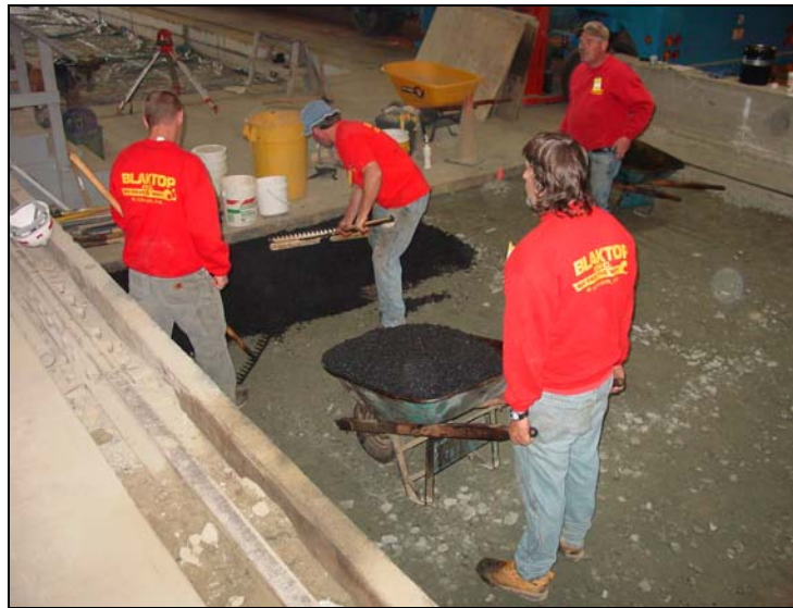
Figure 26. Hand placement of asphalt near the north edge of the test basin.
