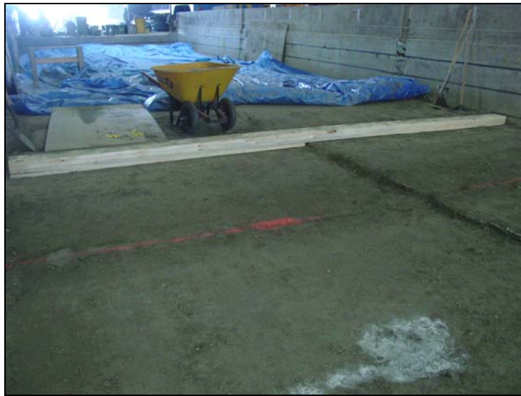
Figure 18. Differences in elevation of the top of the subgrade between test sections.
