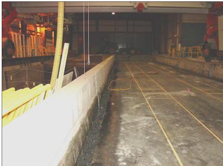
Figure 30. Trench formed by asphalt removal from the edge of the test basin. Water was added to the base layer exposed in the trench to decrease the stiffness of the subgrade layer.
