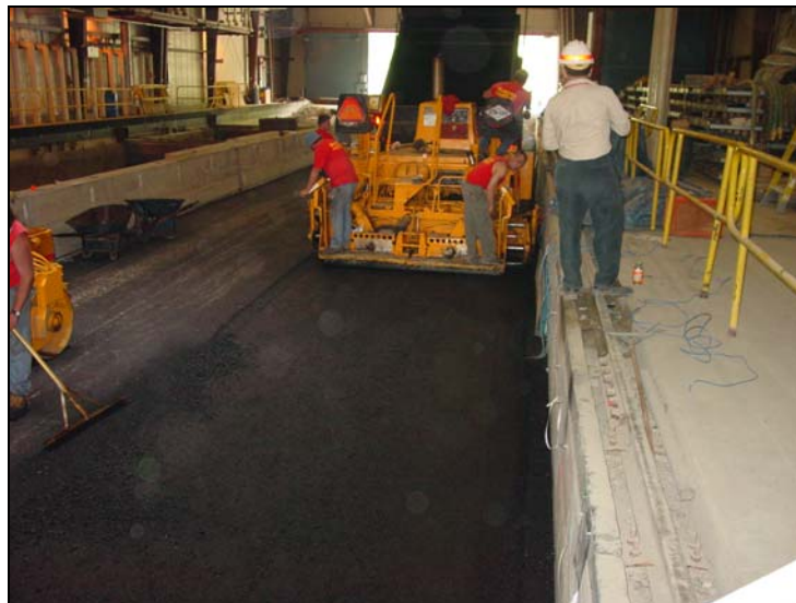
Figure 27. Paving operation during placement of the surface course of asphalt. The dump truck containing the asphalt concrete is in the background, and the paver is shown in the middle.
