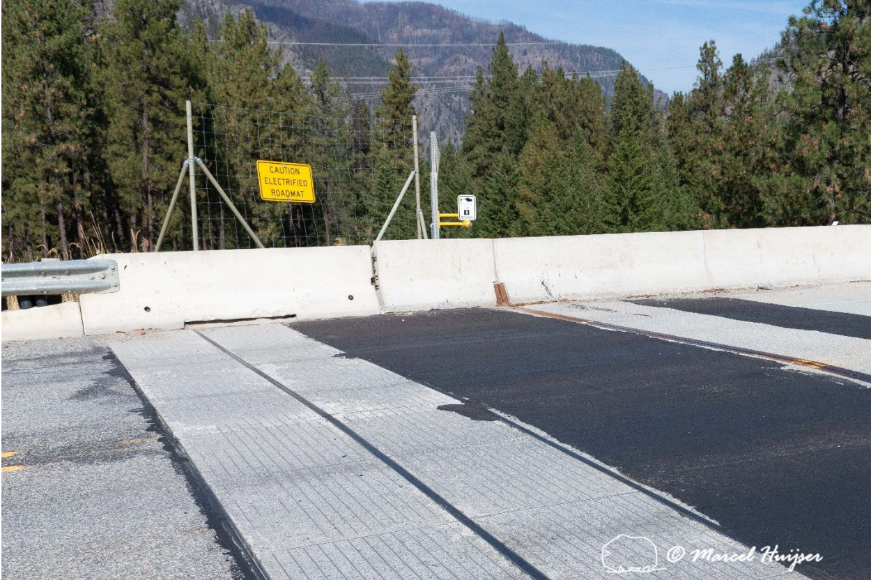
Figure 38: The crumbling concrete at the western electrified barrier was covered in asphalt.
