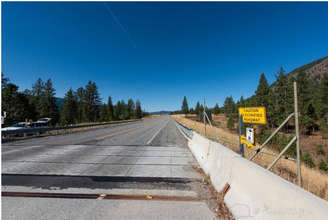
Figure 32: The electrified barrier at the west fence-end. Note that the bridge directly connects to the electrified barrier.
