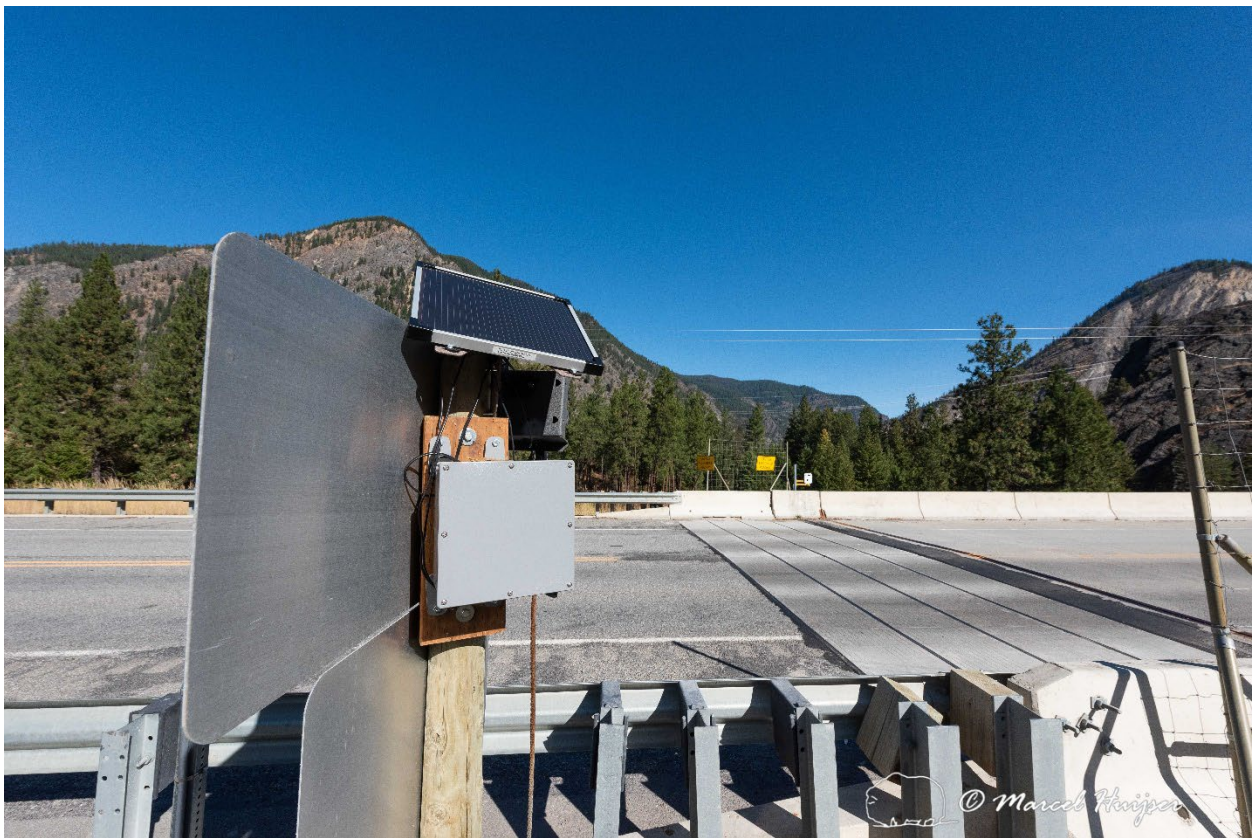
Figure 35: The camera, battery box and solar panel installed on a sign post behind the sign at the western electrified barrier.
