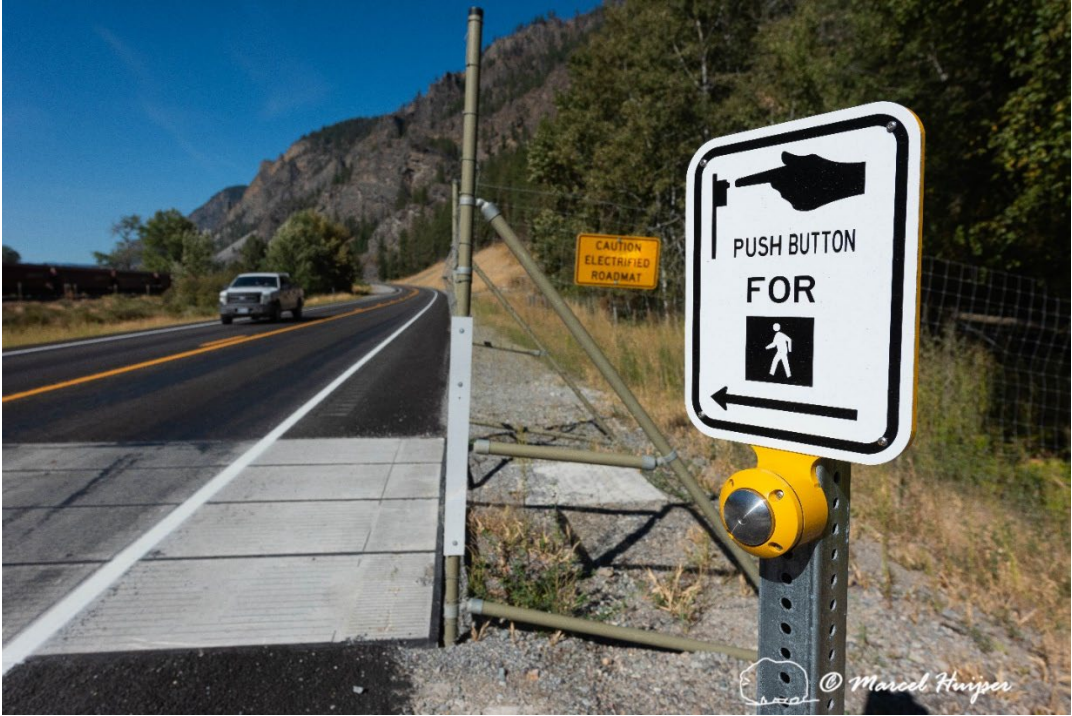
Figure 34: One of the push buttons for pedestrians at the electrified barrier at the east fence-end. There are 2 push buttons; one for each travel direction.
