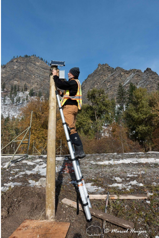
Figure 36: The camera, battery box and solar panel installed on a designated newly installed post at the eastern electrified barrier.
