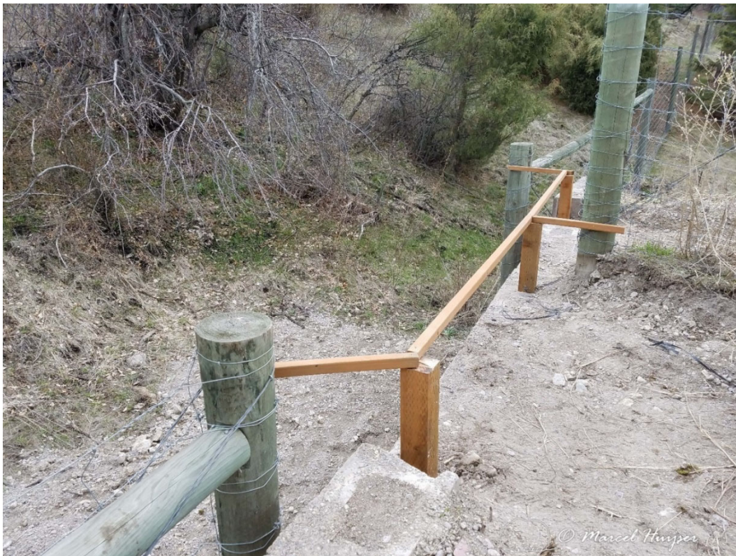
Figure 5: The prototype for the “bar” made from “2x2” inch and “4x4” inch treated lumber.
