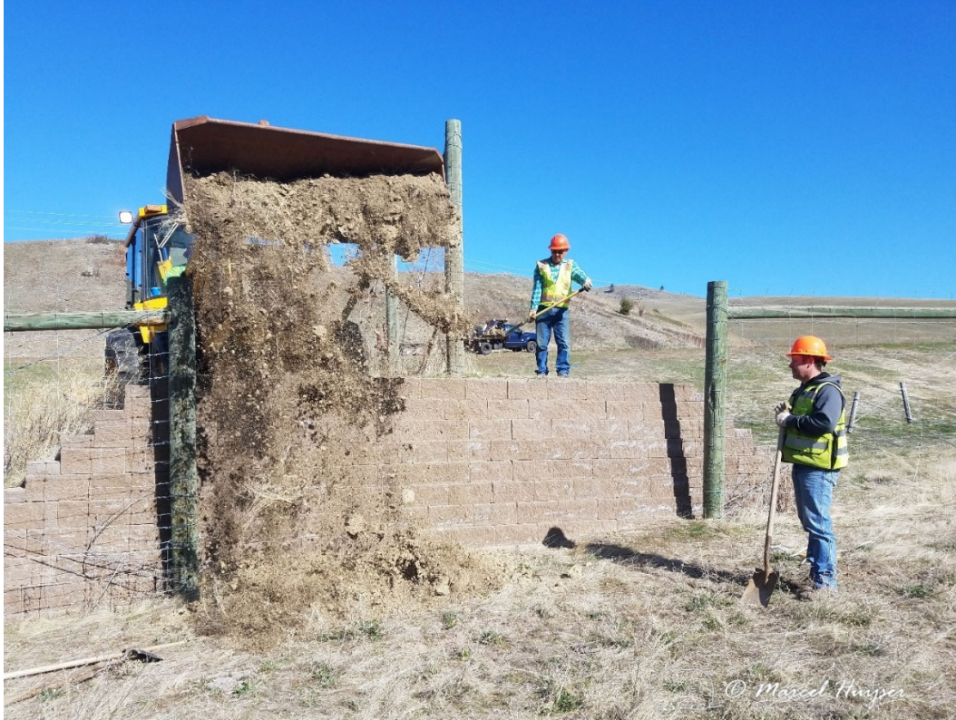
Figure 4: The Montana Department of Transportation assisted with the lowering of 10 jump-outs. After removing concrete blocks of the face, soil from the top was deposited at the bottom for the landing area.
