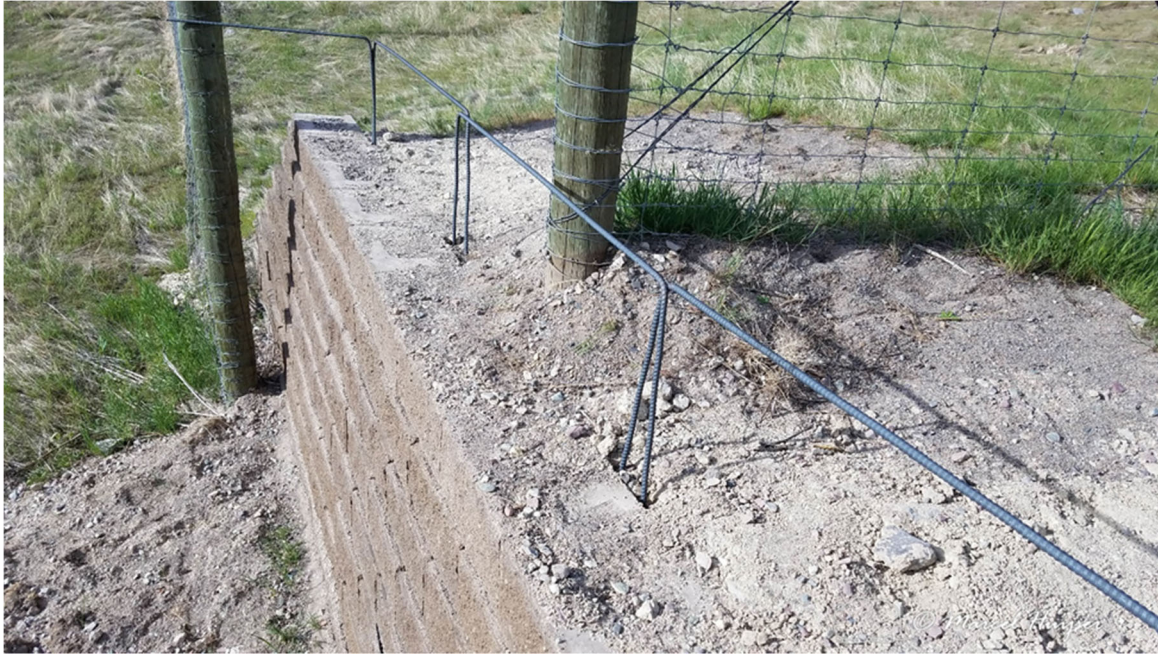
Figure 11: The rebar had a minimum setback of 12 inches (30 cm) as the legs had to be positioned behind the concrete blocks of the face of the jump-out.
