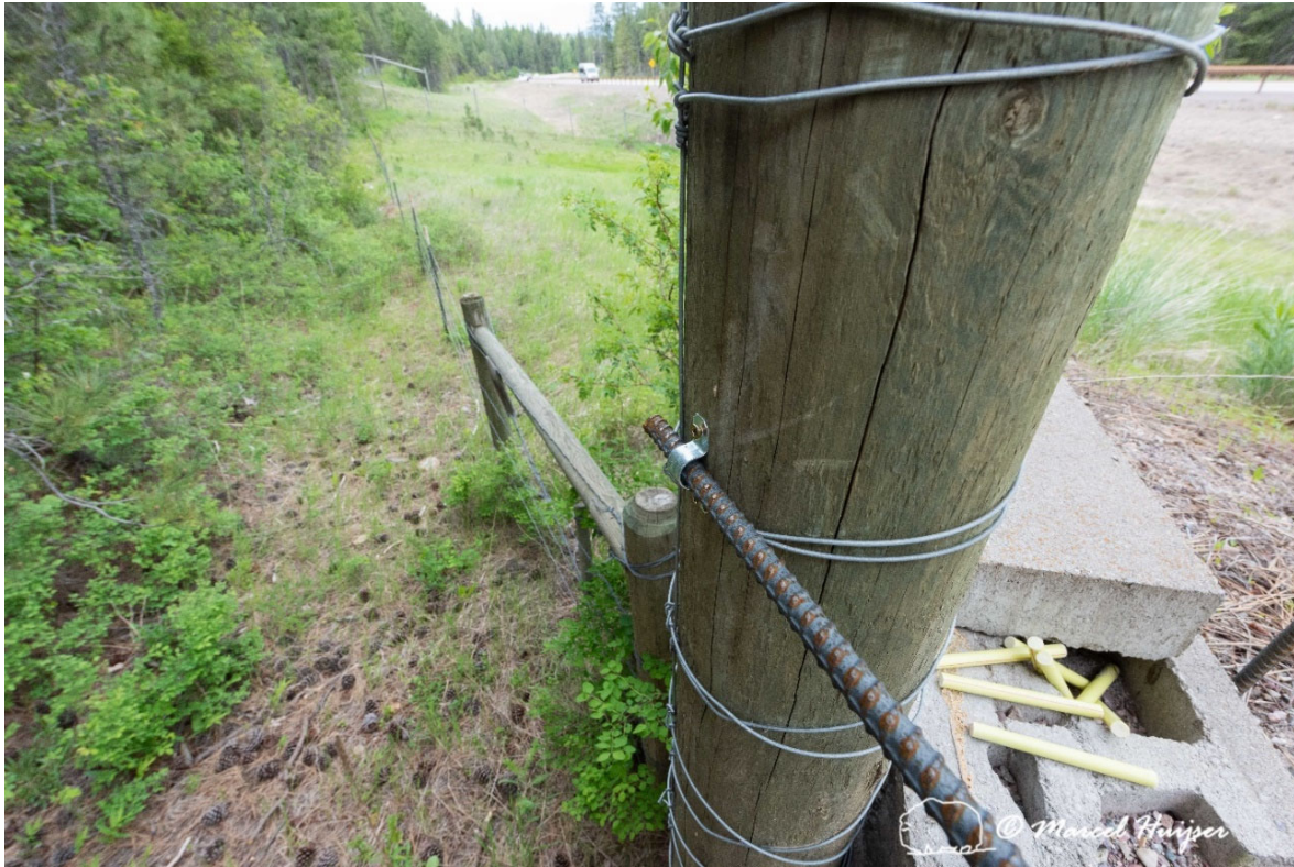
Figure 8: The L-shaped corner elements were connected to the fence posts with brackets and screws.
