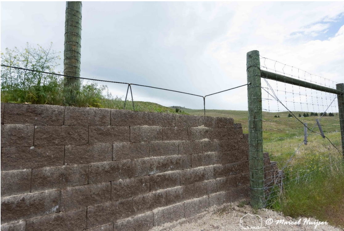
Figure 7: The rebar installed with the L-shaped corner elements connected to the fence post.
