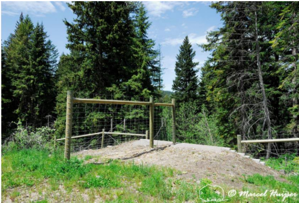
Figure 22. A view of a jump-out on the highway side of the fencing with a perpendicular fence that is designed to direct animals following the exclusionary fence to use the jump out
