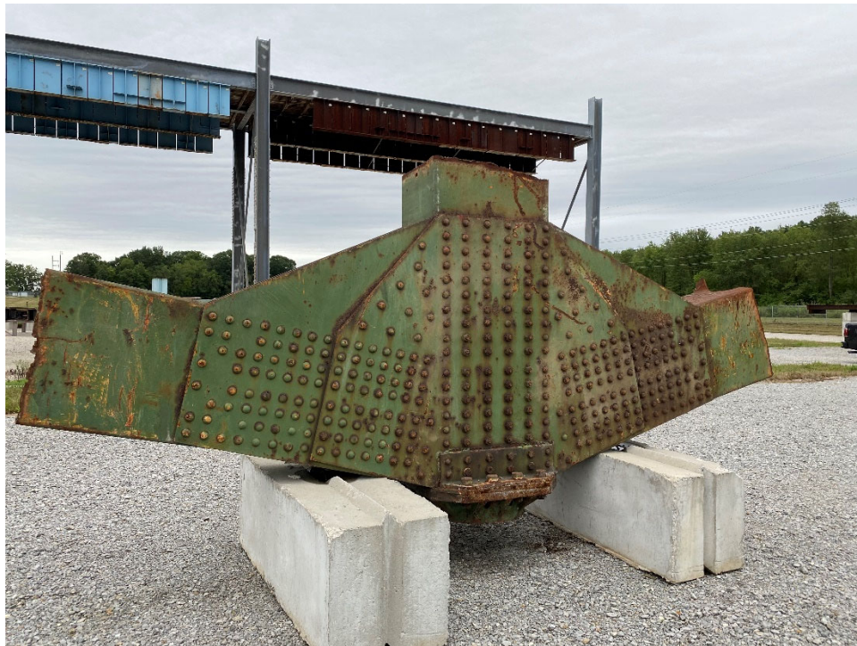
Figure 2 – Photograph of L8 joint from I-35W bridge obtained from FHWA
