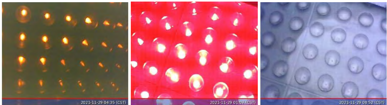
Figure 30: Michigan field test data collected in November 2021 after the field installation on November 4 th , showing the normal performance of the red, yellow, and green signal lights under mild and cold weather conditions. Note that before Nov 17, 2021, the green signal light had a higher lens surface temperature due to its longer power-on timing than the red signal light. This timing sequence was changed after Nov 17 per our request to keep the green and red signal with well-balanced power-on timing, resulting in close temperature measured on the lens surface for both green and red light.
