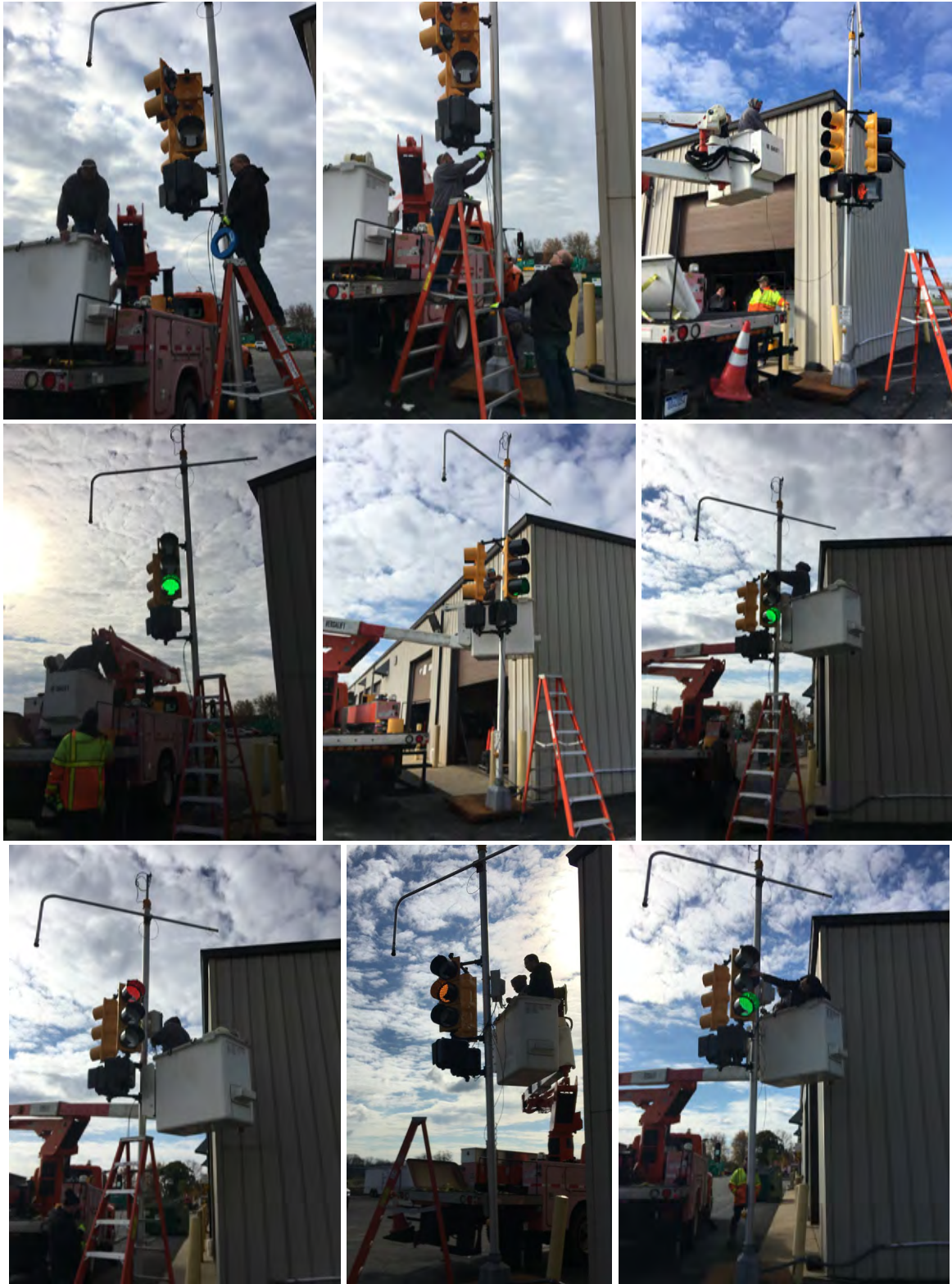
Figure 29: Field installation and setup of the onsite testing at the test site of Michigan in front of the signal shop, with the aid of the signal crew of Michigan DOT. A tunnel visor was installed with hook for mounting the cable camera on each signal module. The signals are facing north.
