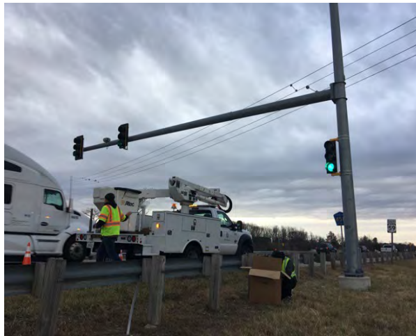
In preparation, the existing LED signals
