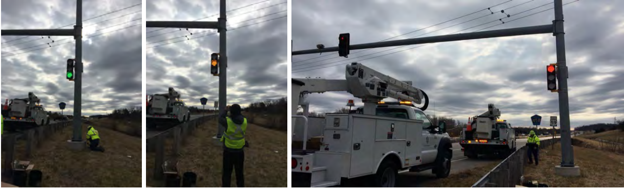
New green /orange signals are powered on
