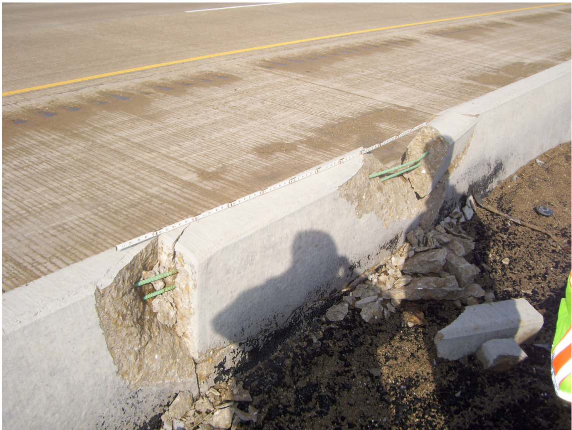
Figure 4. Cracking of Concrete Barrier
