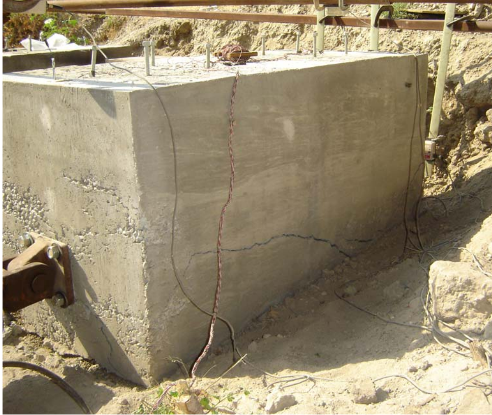
Figure 7 Initial cracking Test Cap 3.
