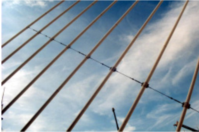
Figure 11: Cable cross-tie system.
