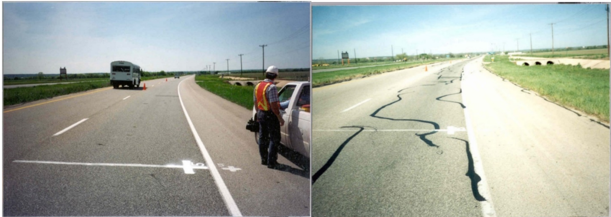
Figure 14. Test section at Station 5+00 looking westbound in 1993 (left) and 1995 (right) depicting an increase in crack sealing during this period.
