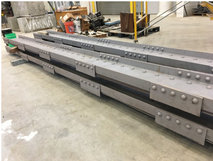
Figure 2 - Members ready for shipping to fabricator after sandblasting. A web and top flange will be added so these former lower chords can be loaded in flexure.
